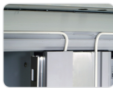
Heating cable to prevent ice build-up
